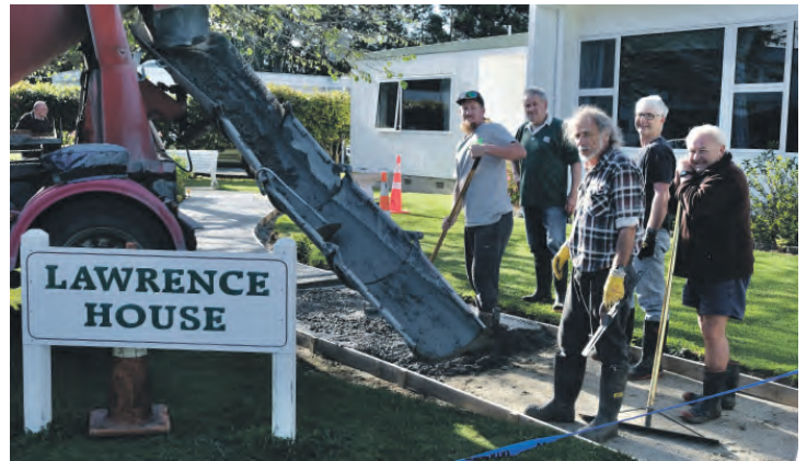
ABOVE: Bowers Concrete donated the concrete to lay a new path at Lawrence House. Photo by Peter Kampenhout.
